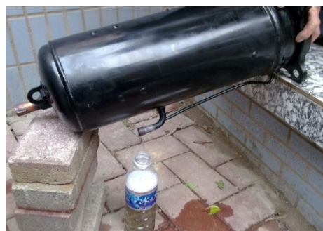
Figure 6-2.8: Draining oil from a compressor
