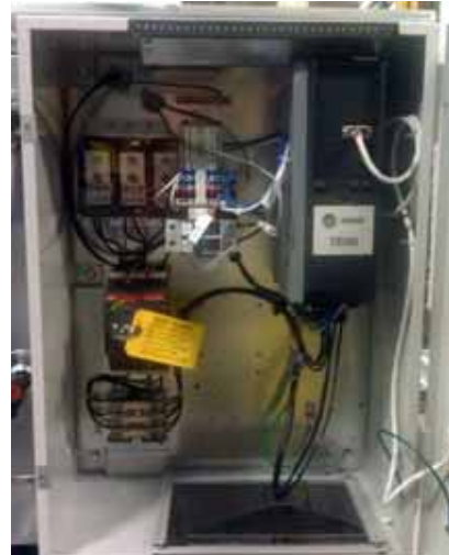
Figure 147. Externally mounted VFD
