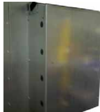
Figure 151. Externally mounted control box
