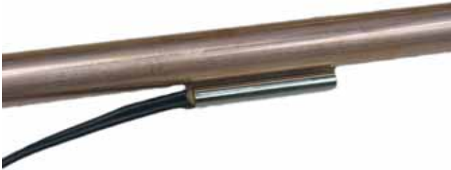
Figure 31. Close-up view of the entering water temperature sensor
