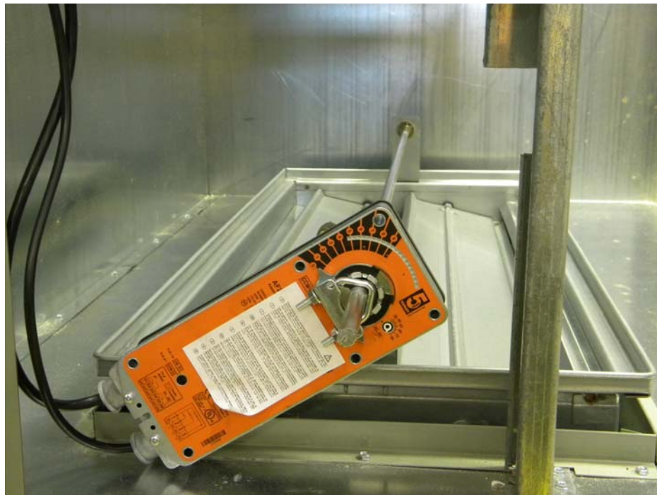
Figure 63. Return air damper
