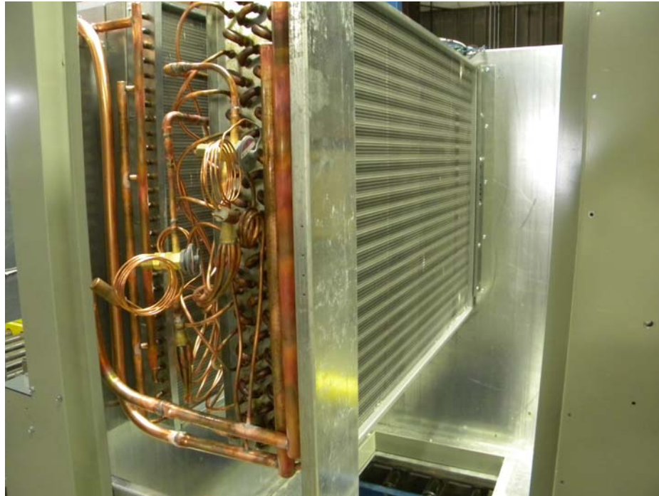
Figure 59. Evaporator and reheat coil
