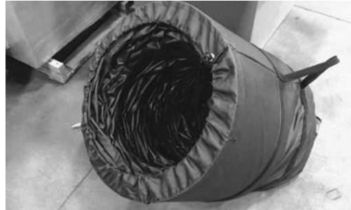
Figure 10. Collapsed 20 in. duct
