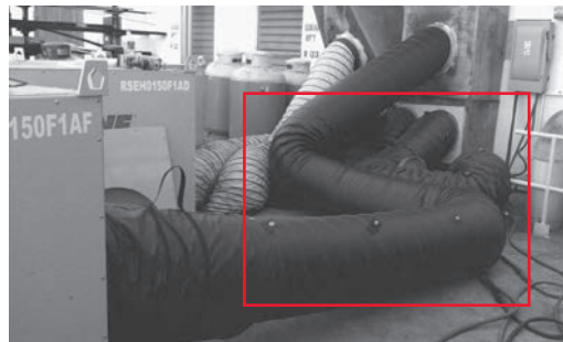
Figure 11. Flexible duct connection
