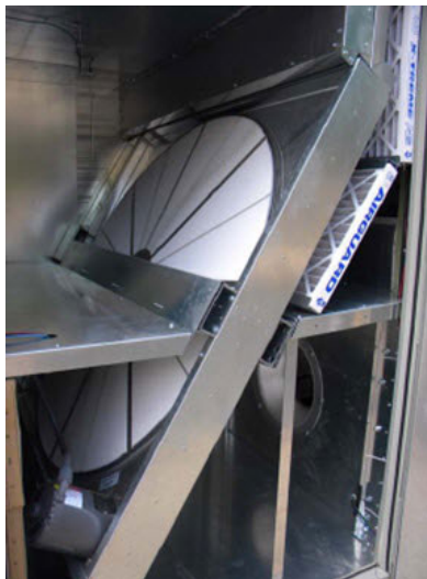
Figure 47. Total-energy wheel inside a dedicated outdoor-air unit
